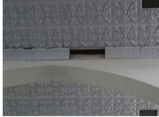
Fig. 1.8- A part of false ceiling fell off due to earthquake
