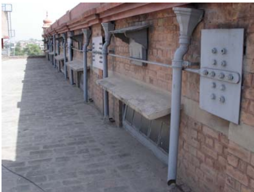
Fig. 1.5- Improper drainage on the roof of the main building
