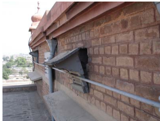
Fig. 1.6- Rain water can penetrate in the ceiling through roof windows
