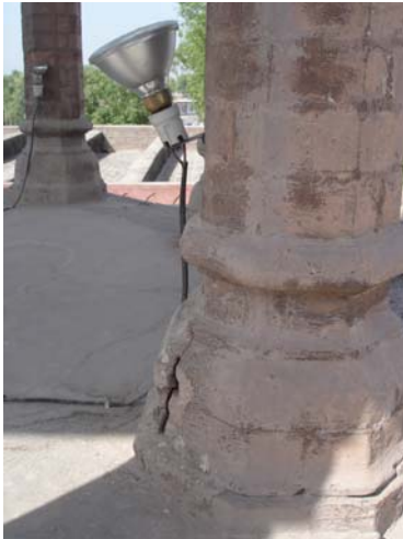
Fig. 1.3- Damage to roof cenotaph due to October 2005 earthquake
