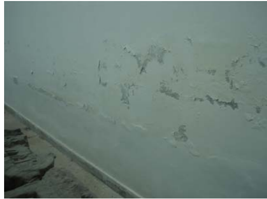
Fig. 2.8- Dampness can be seen on the walls of the storage.
